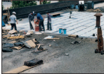
Unnecessary Roof Repair
