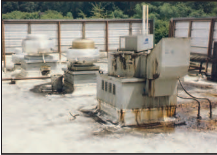
Grease Laden Rooftop
